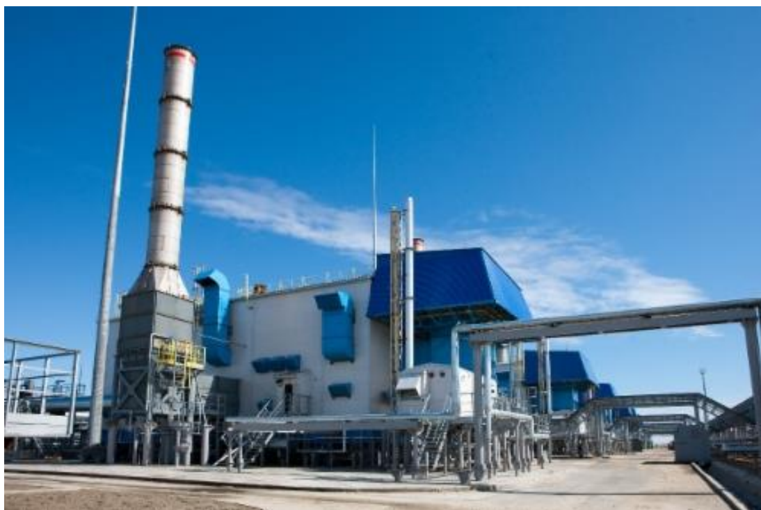
Figure 4-6: Example for a compressor station (Baidaratskaya compressor station) (Gazprom, 2016)
